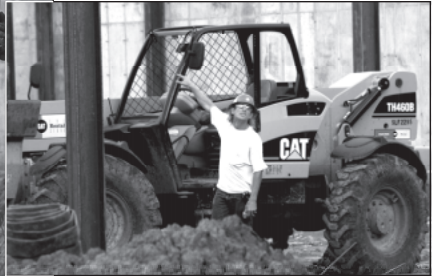
Mark Dewarns of All Steel Building Co. gives directions to the crane operator for placement of the next steel support. Crews work swiftly between rain delays to keep the construction of the new Health Professions Education Center on schedule.
